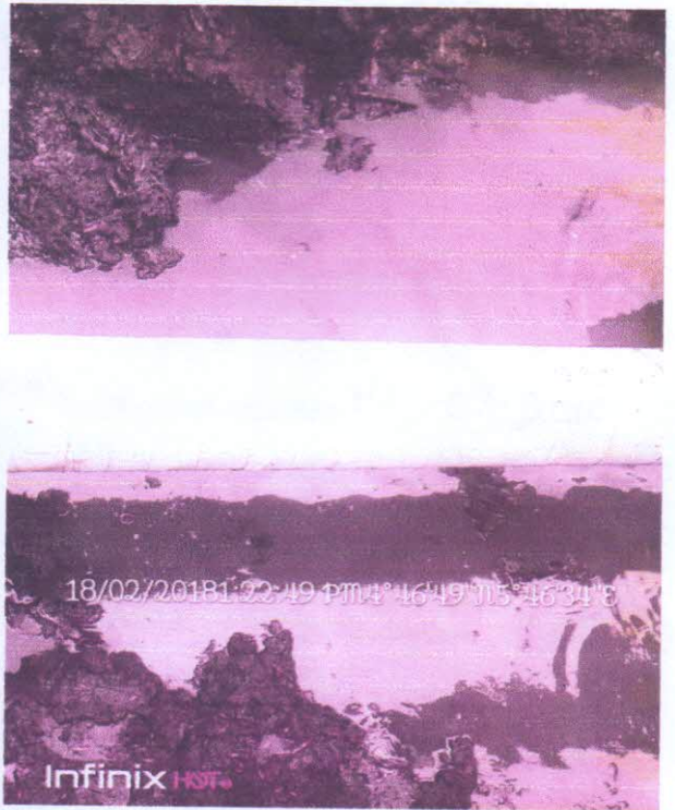
LEAK POINT AFTER REPAIR
